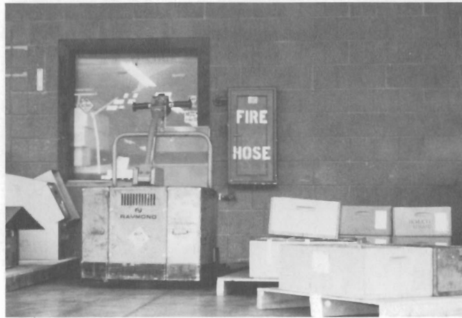
blocked firefighting equipment ...
